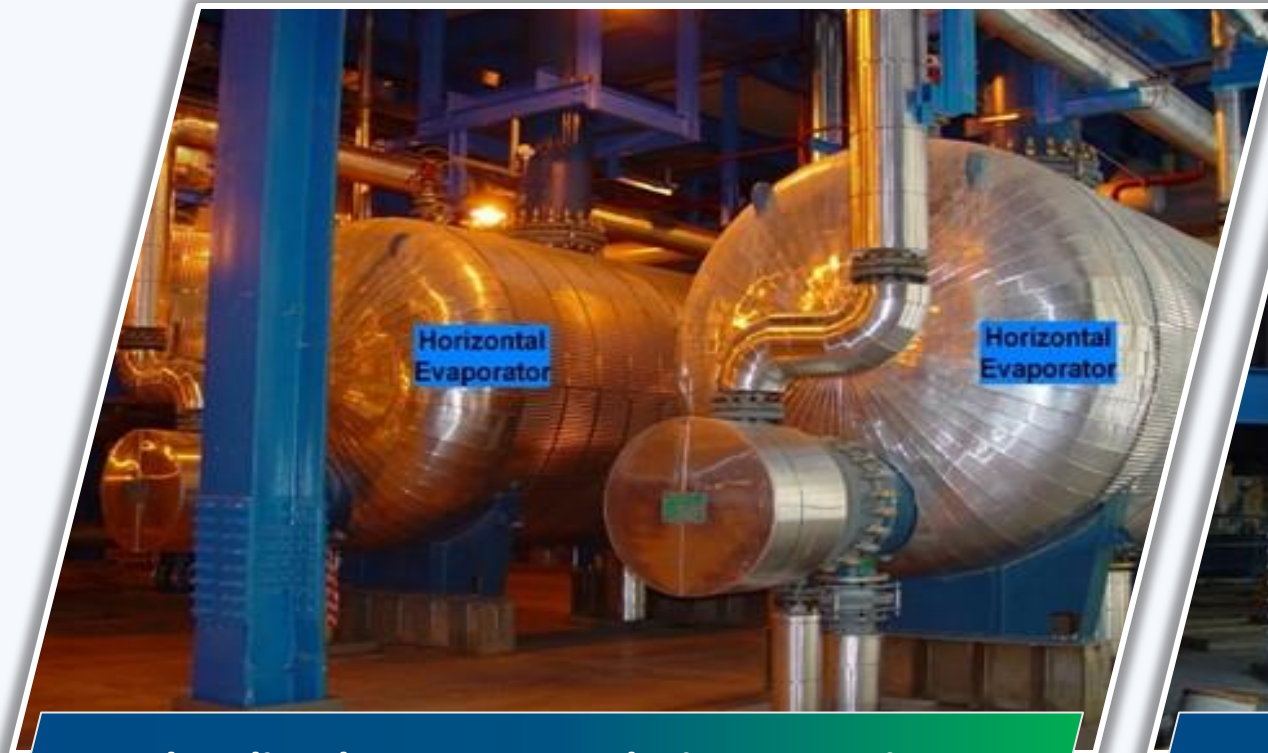
Glass lined evaporators during operation (insulated)
