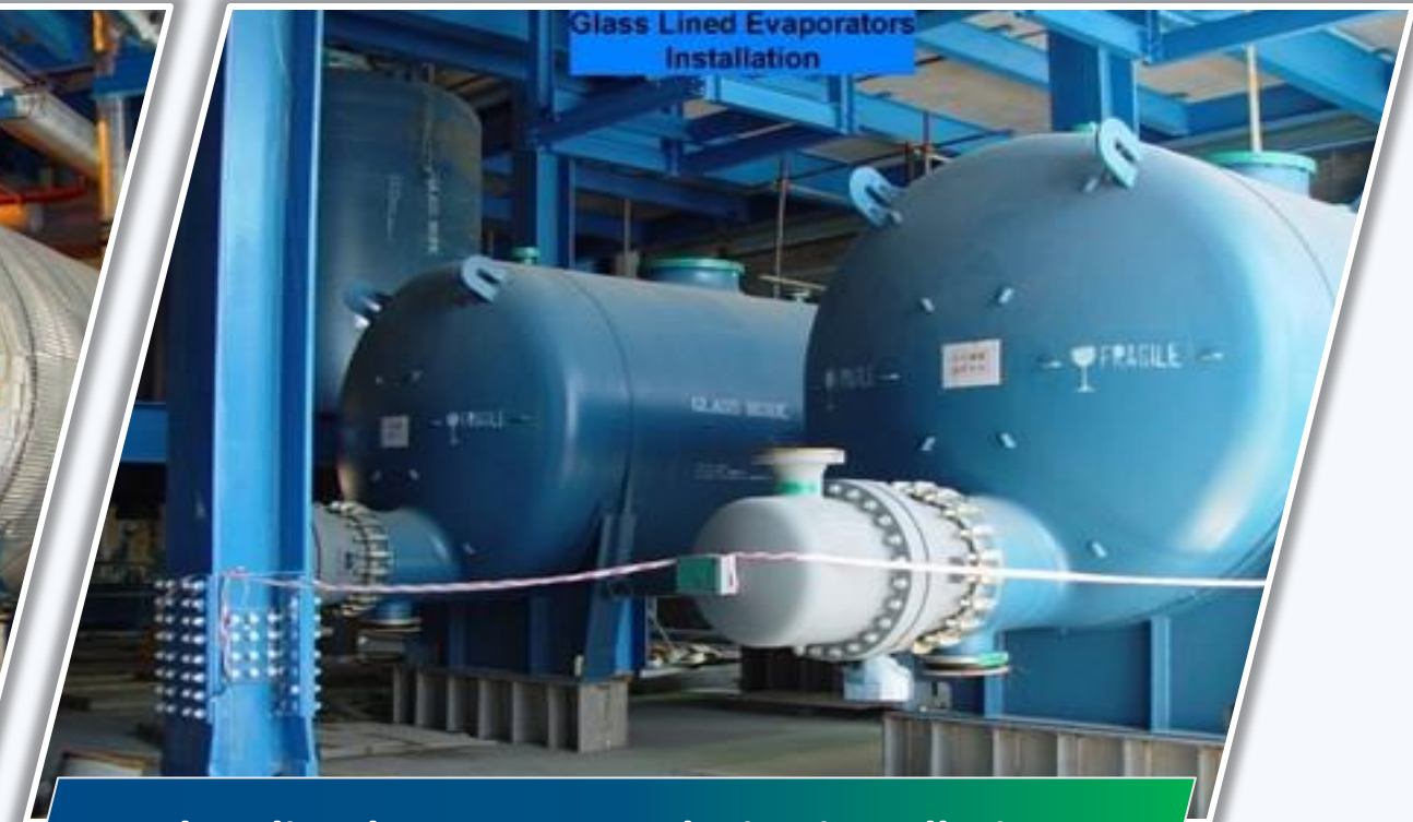
Glass lined evaporators during installation (non-insulated)
